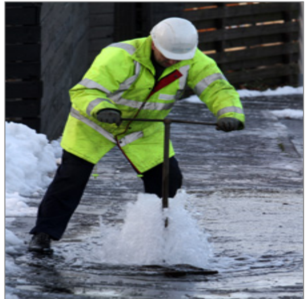
Above is a Scottish Water worker dealing with burst water main
