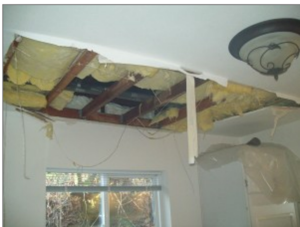
Partially collapsed ceiling
