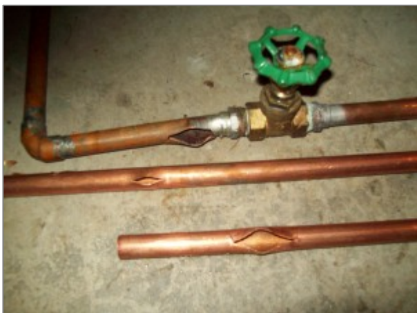
Burst copper piping due to freezing
