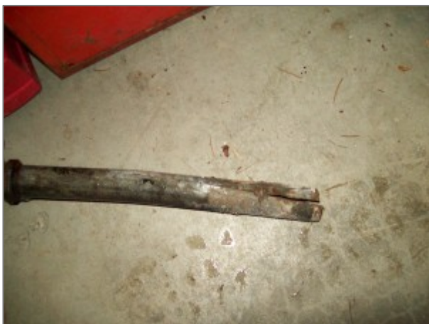
Cracked galvanised piping due to freezing
